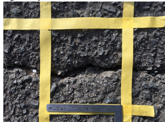
Fig. 8 Picture of rough surface road with complex crack.
