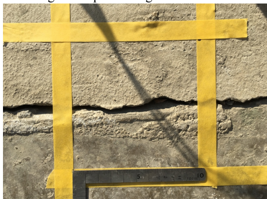
Fig. 6 Picture of smooth surface road with straight crack.
